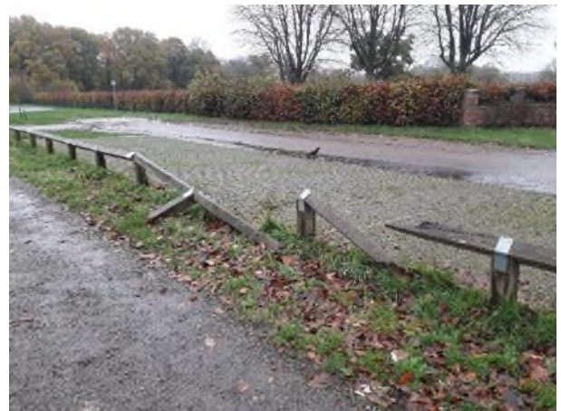
Damaged kick rail fence in the main car park
